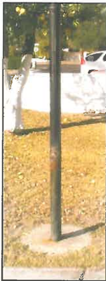
Photo 4a. External Rust On Second Exemplar Pole
