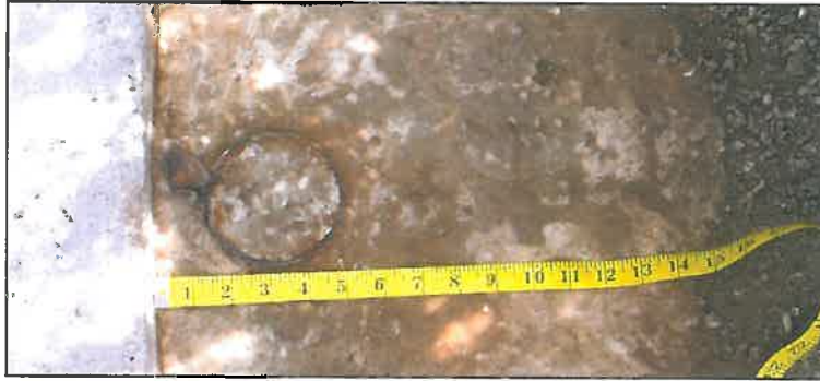
Photo 7a. Corroded Pole Stub In Desert Landscaping
