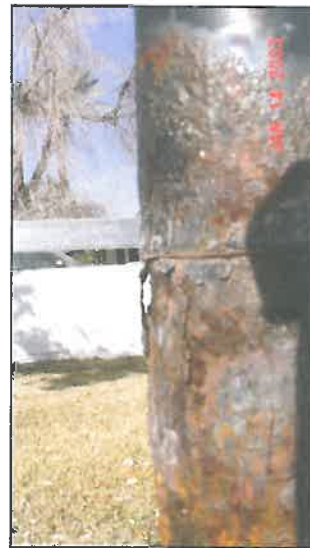
Photo 4b. Layers of Rust, Pushed Away From Pole Metal At The Joint Between The Lower And Middle Sections Of The Pole
